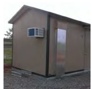
Electric Sub Station
