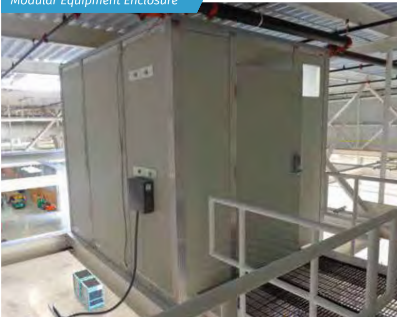
Modular Equipment Enclosure
